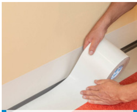
4. Placement of a new strip of Mapecontact Plus on the floor by overlapping the cove former slightly
